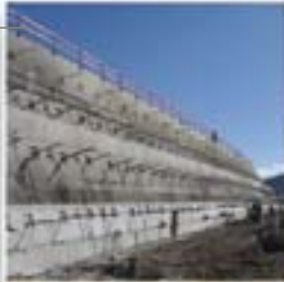
■ Anchored walls at Troinex on the A41N highway (France) Advisory services to client
