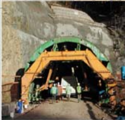
■ «Pont de l'Eglise» Tunnel in Reyvroz (France) Detailed design and construction drawings
