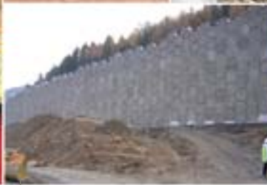
■ Coynelle section of the A51 highway, Col du Fau (France) Detailed design and construction drawings
