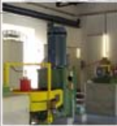
■ Turbo-generator set of Vessy hydro- power plant (Switzerland) Design and project management
